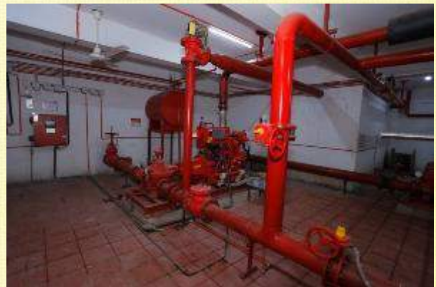
Fire Pump Station
